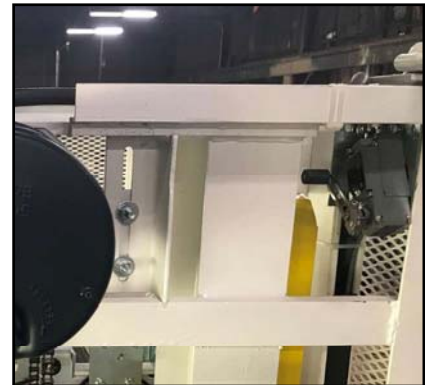
Inspect Limit Switch Arms Figure 21-2
